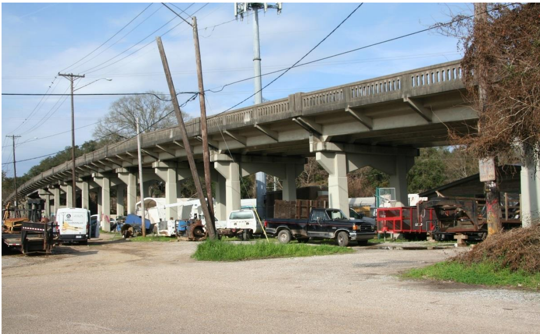
Character-defining Feature Photo 2: Design and construction of a railroad grade-separation overpass. The steel I-beam span, which crosses the railroad, and adjacent concrete deck girder spans comprise the superstructure.
