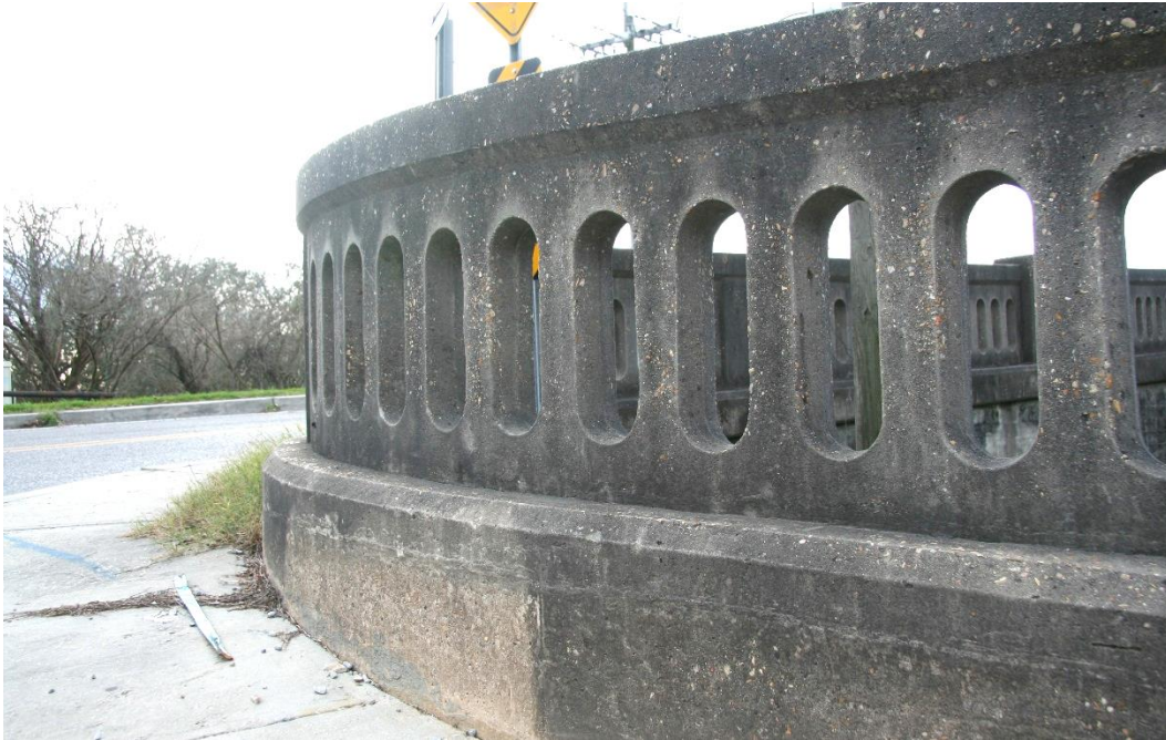
Character-defining Feature Photo 3: Aesthetic treatment of decorative open balustrade railings conveys the bridge's architectural significance.
