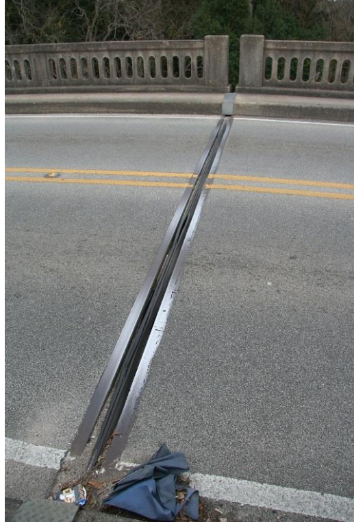
Condition Photo 11: Roadway expansion joint near Pier 7 at steel beam span over railroad.
