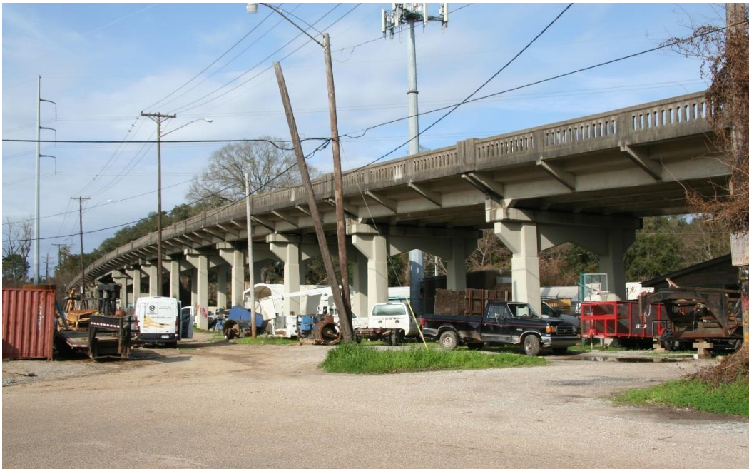
Condition Photo 2: View of west elevation of bridge. Note coating of piers from 2009 rehab.
