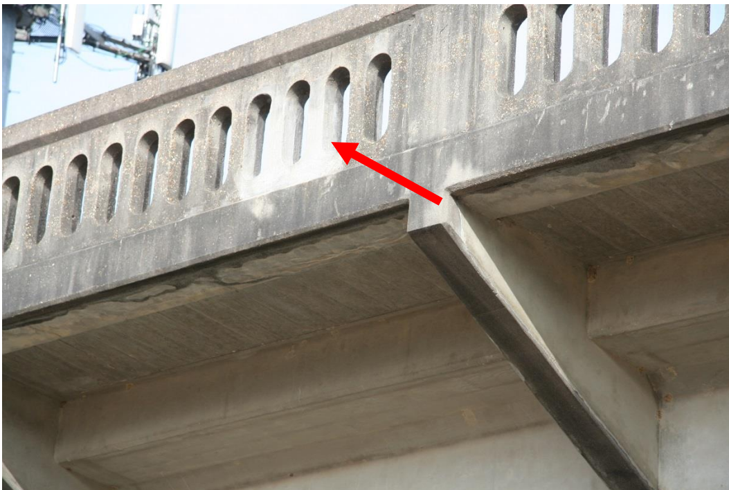
Condition Photo 4: Repair of section of bridge parapet. Note variation of concrete color and texture.
