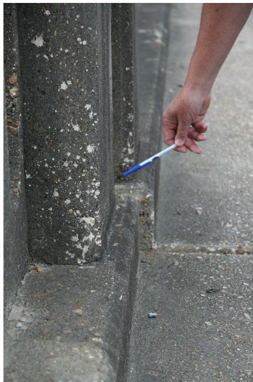
Condition Photo 12: Approximately 1-inch offset between parapets and deck at pier 8 (spans 7 and 8).
