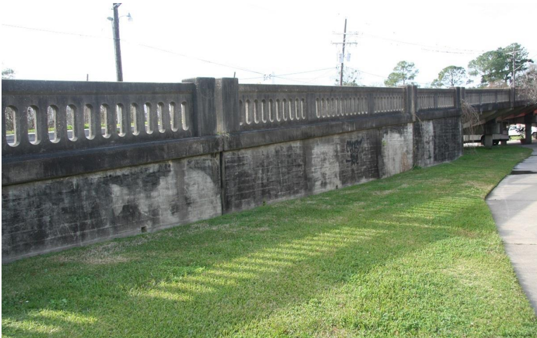
Historic Fabric Photo 1: Concrete retaining wall at the southeast corner of the bridge.
