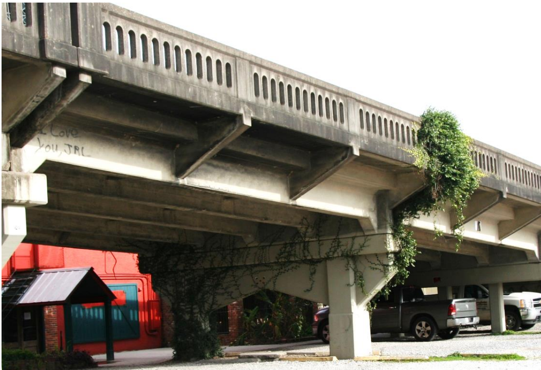
Condition Photo 8: Vegetation growing on pier and superstructure.
