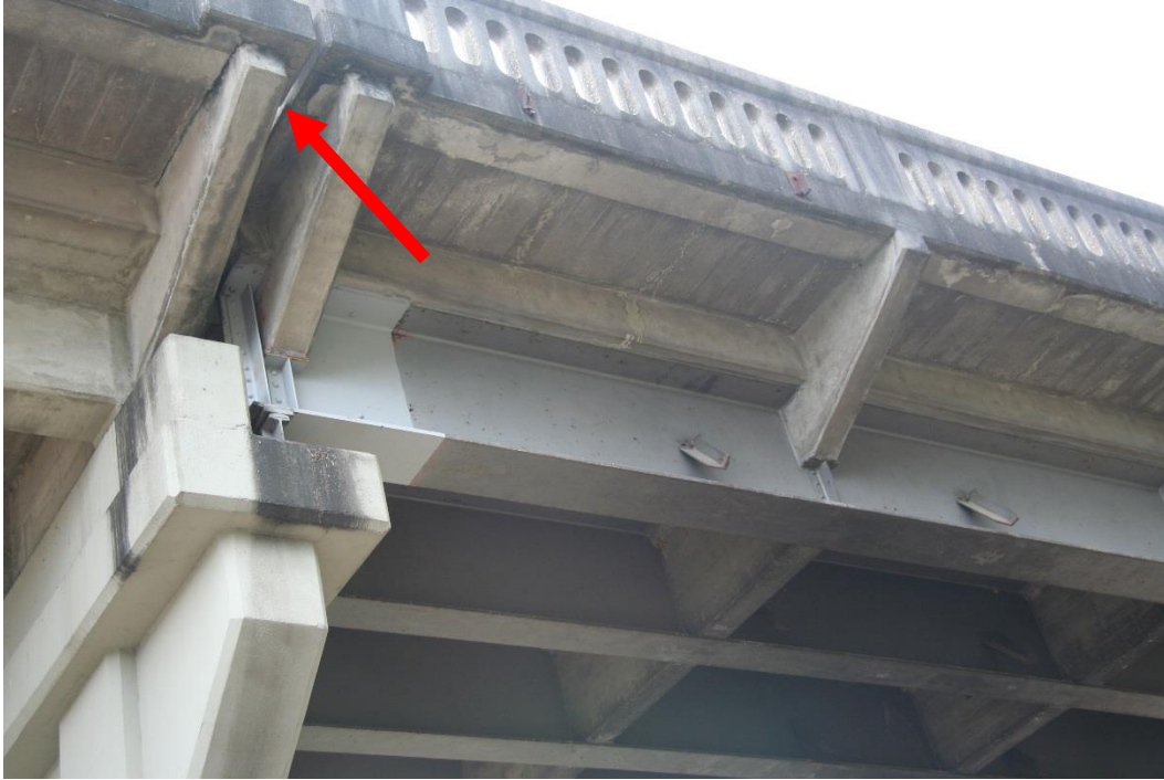
Condition Photo 7: End of steel beam span at pier. Note additional painting of ends of steel beams, expansion joint in deck above, and two remaining steel angle members attached to the beam from the removed metal blast plates and their supports.
