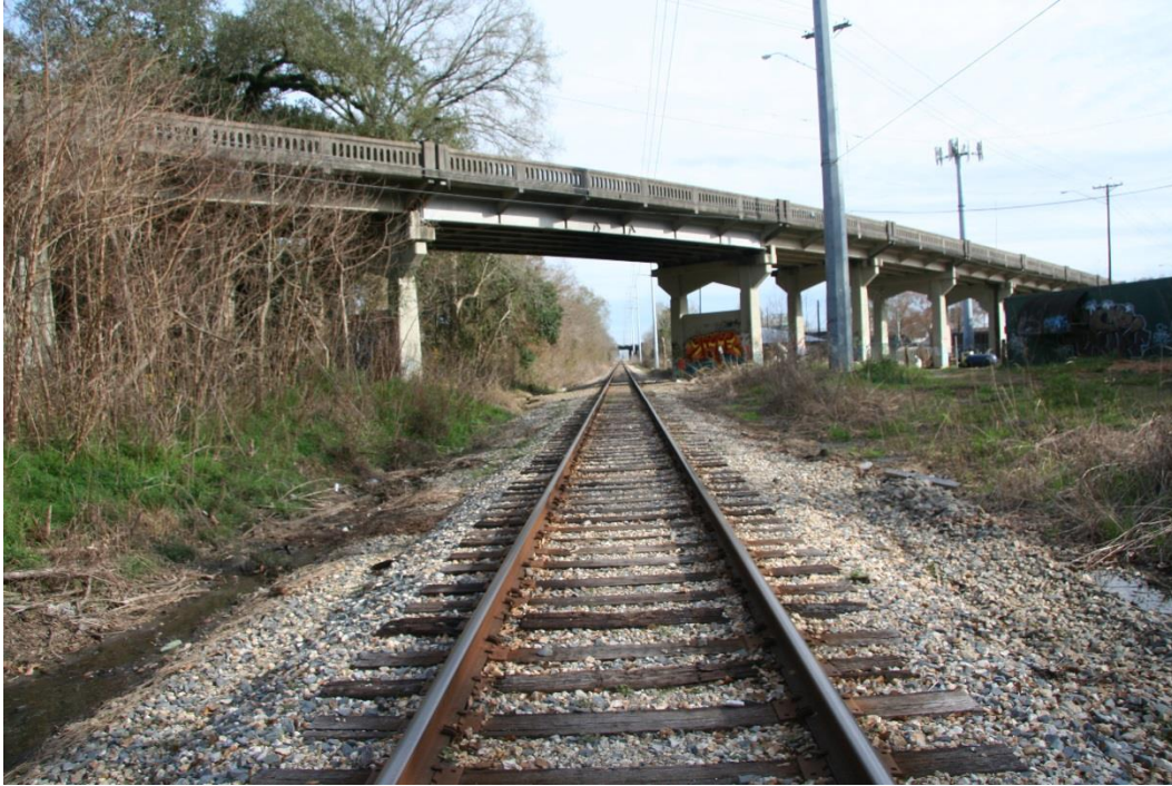
Character-defining Feature Photo 1: Design and construction of a railroad grade-separation overpass. The steel I-beam span, which crosses the railroad, and adjacent concrete deck girder spans comprise the superstructure.
