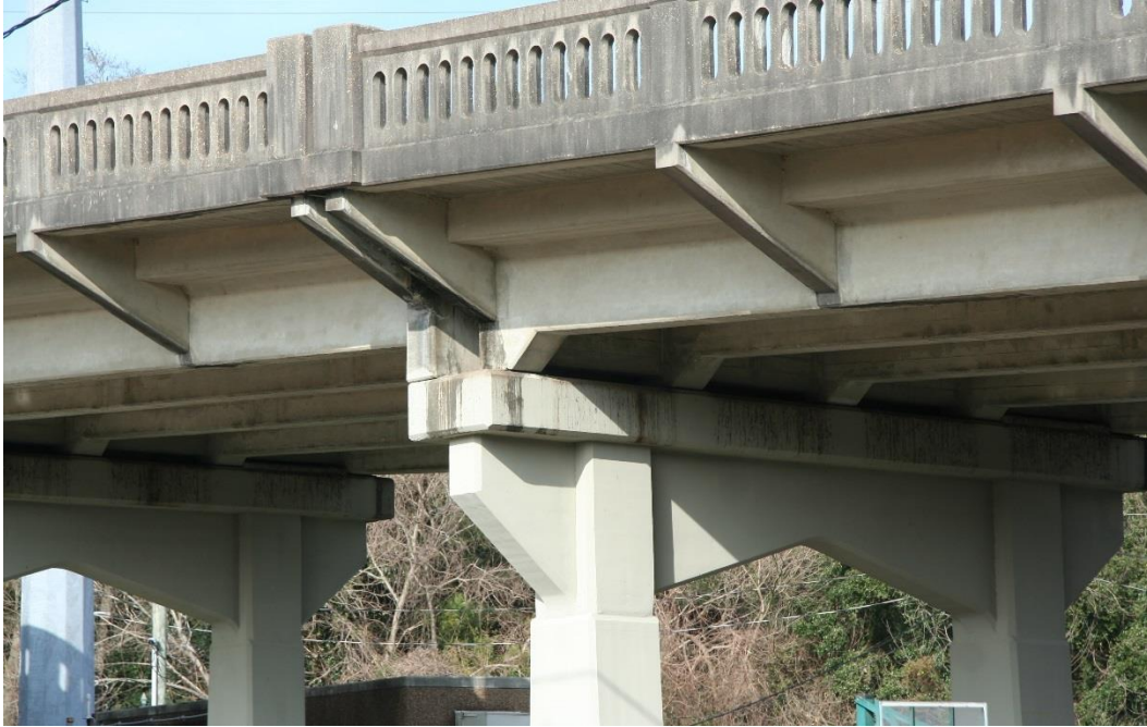
Character-defining Feature Photo 5: Aesthetic treatment of brackets supporting the cantilevered sidewalk and angular pier caps demonstrates the architectural features of this bridge.
